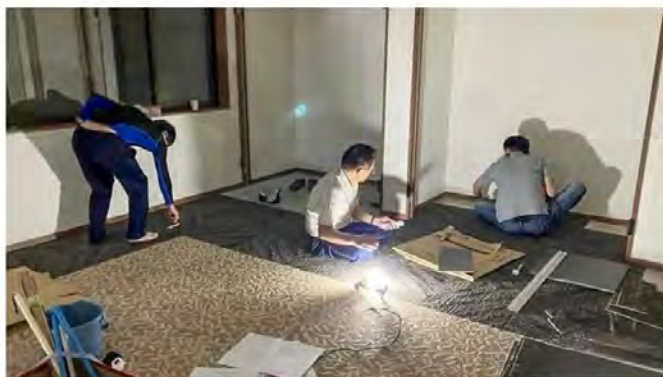
Believers of the Family Federation’s Koriyama Church tiling during construction of the new church facility. Photo: FFWPU
